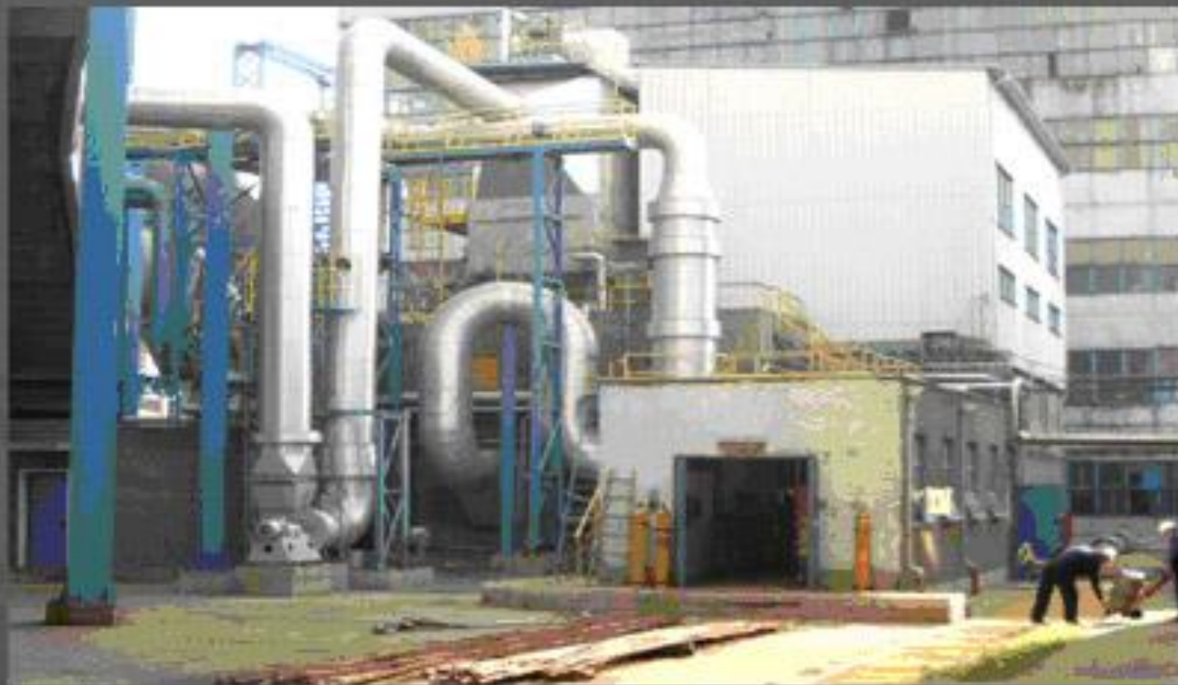
Electron beam plant –common view
